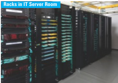
Racks in IT Server Room
